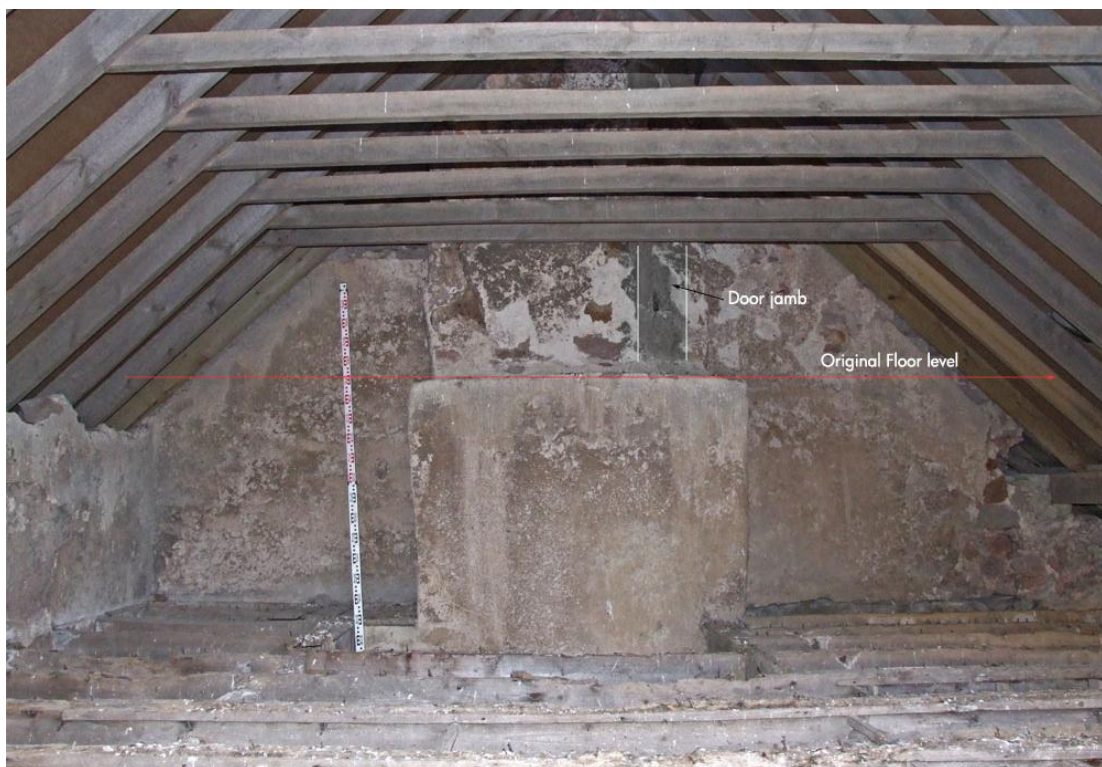
Plate 7: Room 18 roofspace with original floor level for the second floor marked and the original doorjamb highlighted.
